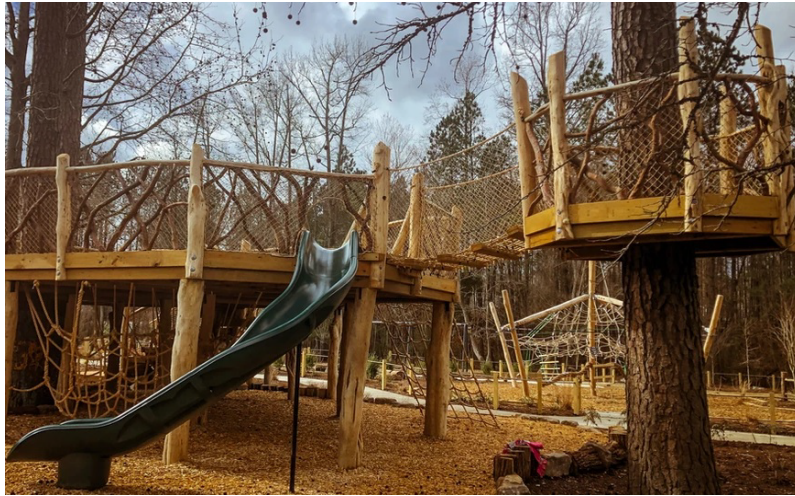
Deck/train tracks to slide (handrails not on decking)
